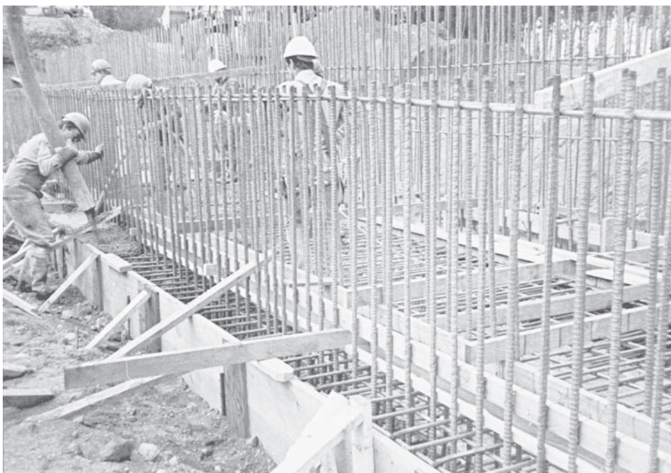
FIGURE 1-4 Concrete construction in progress. Note formwork, reinforcing bars, and pumping of concrete. (George Limbrunner)
